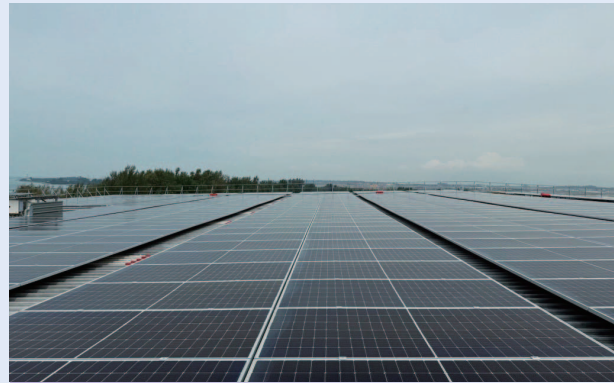
Newly installed photovoltaic panels at 51 Alps Avenue
