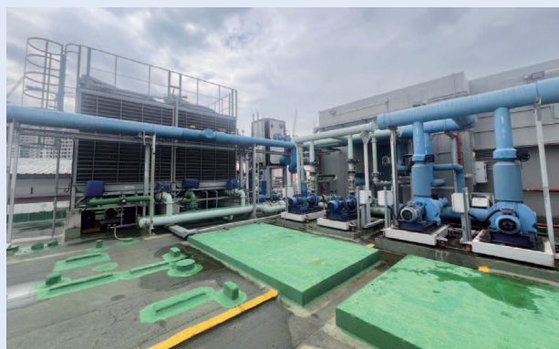
Energy efficient water-cooled chiller system to be installed by tenant
