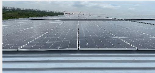
E-LOG is on track to achieving its target to achieve 50% increase in solar power generation by 2025 (from base year 2019)
